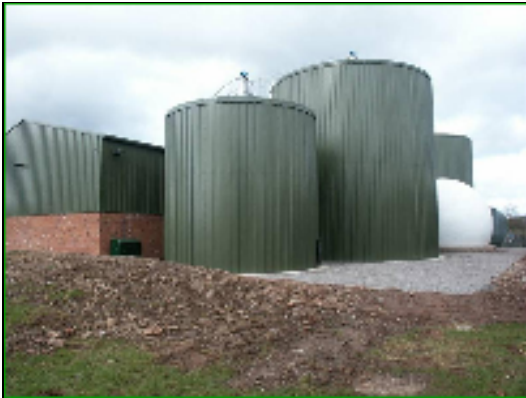
Above - Photo of an AD facility
